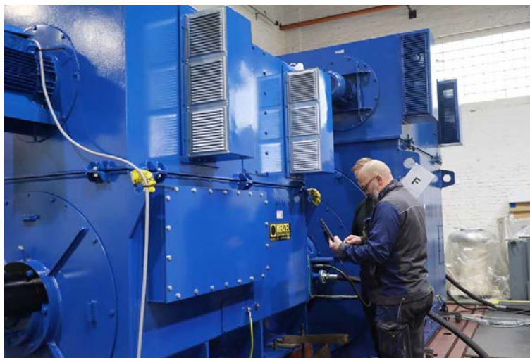
Caption: Menzel manufactured the motor and generator and planned the complete rotary converter set for measuring and testing power transformers
